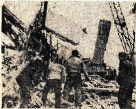
Huge cranes remove concrete slabs that used to be part of the J. C. Penney store in downtown Anchorage.
