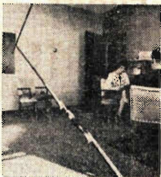
Many Anchorage offices that escaped destruction look like New York life's, where steel braces are welded to pillars to help prevent further shifting of the building.
