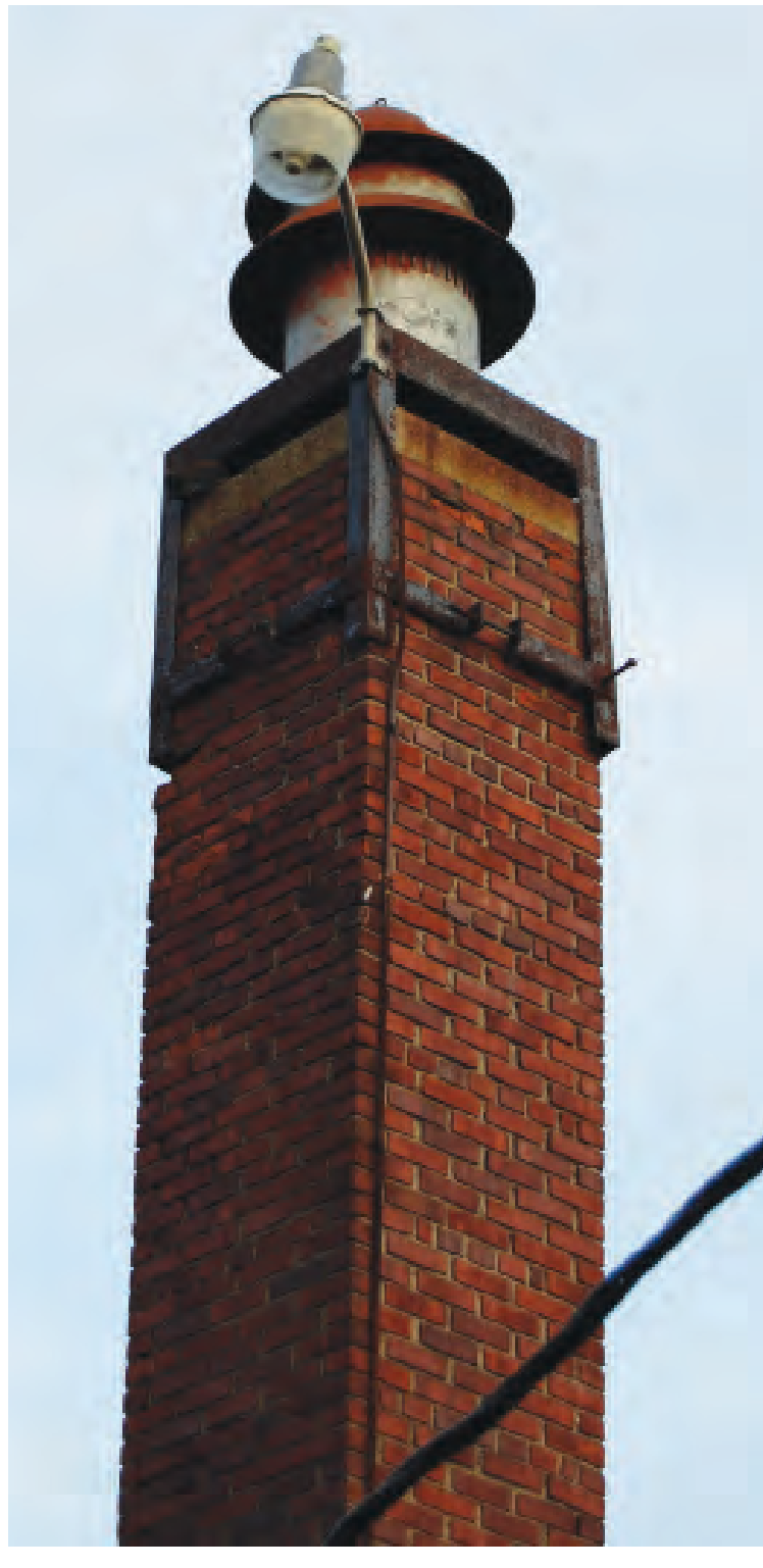
For over five decades, this chimney has been home to the siren seen atop it, all on top the town hall building. Today the chimney is deteriorating, causing the town council to move forward with plans to replace it.
