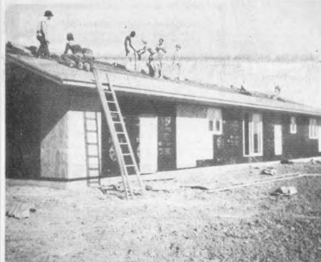
Culver - CCHS Building and Trades afternoon class is shown preparing the home
