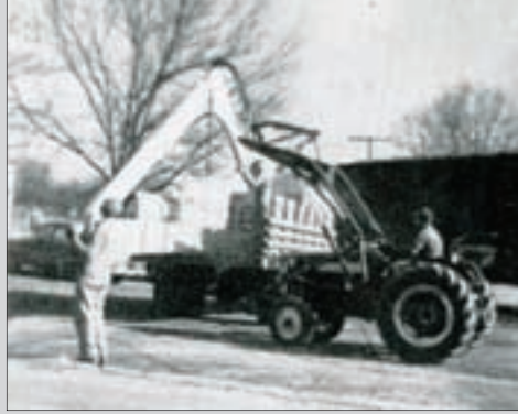
ABOVE: Part of the Culver Bible Church, which had been shipped to town by rail, arrives at its South Main Street location. (left), and the building’s framework rises early in the construction process.
